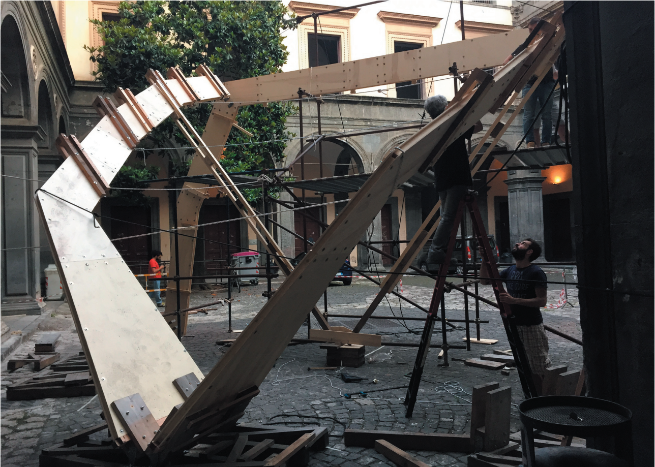
Fig. 8 The arch and the “ribs” of the structure of ReS 4.0, during the building phase in the courtyard of Palazzo Gravina, Naples. Ph. Sofia Colabella.
